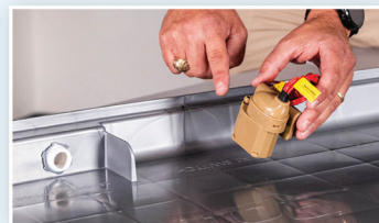
Float Switch Installation
